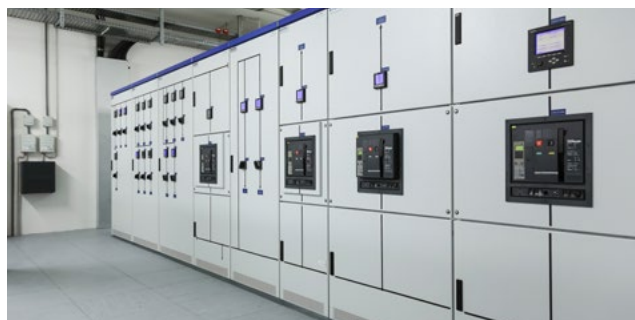
Luxconnect's low-voltage distribution room.
